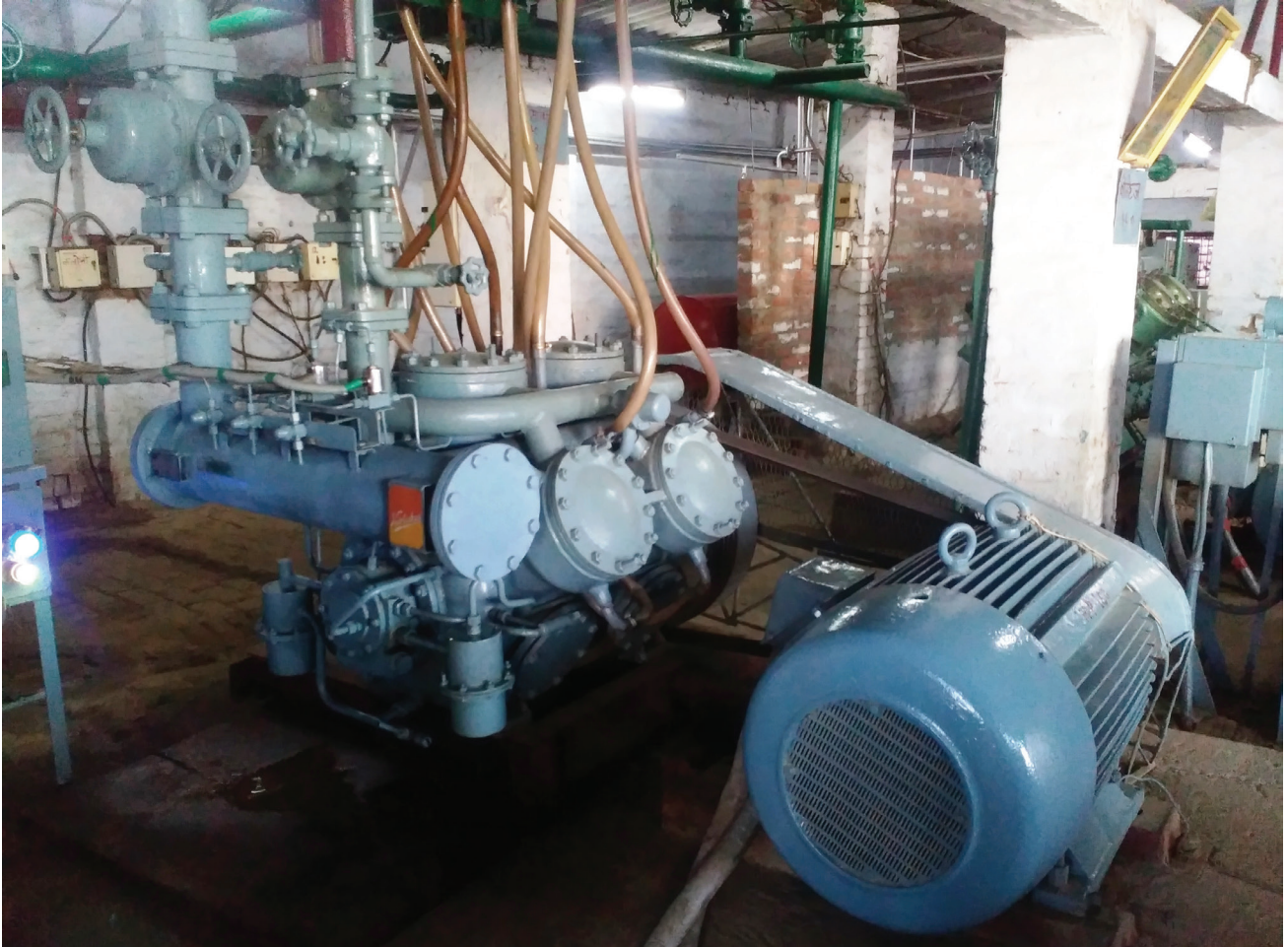
Refrigeration system in cold storage
